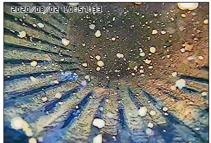
Downhole camera inspection of an observation well showing screen biofouling (2020, WLRS).
