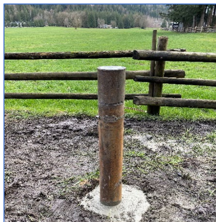
Completed wellhead at OW503 in Chilliwack during March 2022 drilling. Photo credit Ministry of Forests.
