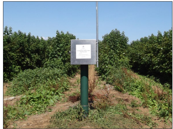
Observation Well #2 in Abbotsford, included in the network since the 1960s. Photo credit: B. Jackson
