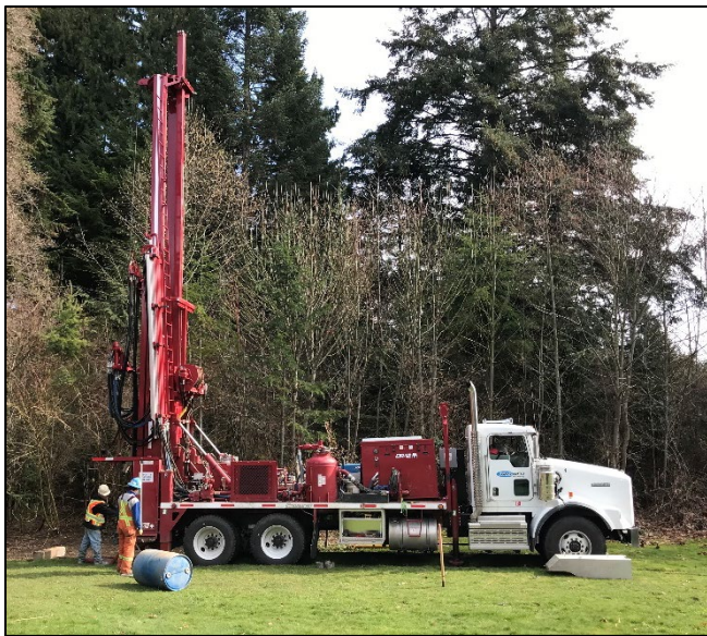
Drilling of OW498, from 2020/2021 Groundwater Compendium Photo credit: B. Jackson, Mission Point Park, Sechelt.
