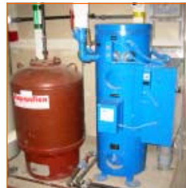
Never used back-up boiler
