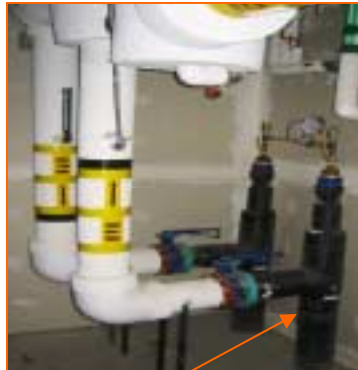
Ocean loop tie-in at mechanical room
